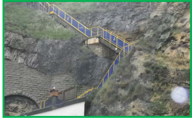
Rockfall protection netting at Marsden Grotto stairs.
