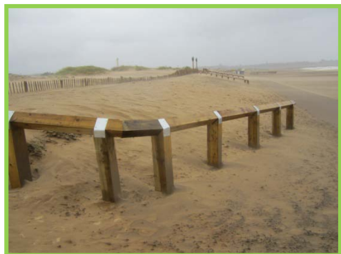
New pedestrian zoning barriers at access points in good condition.
