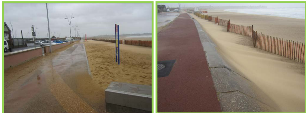
High beach levels, windblown sand on promenade adjacent to Public House. Spalling and abrasion along the sloping concrete revetment.
