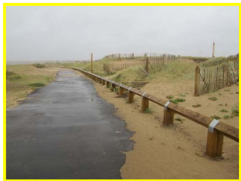
Dune fencing in good condition but 'donkey track' showing signs of distress.
