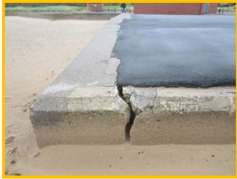
Settlement of the promontory area and wide cracks in the reinforced capping beam.
