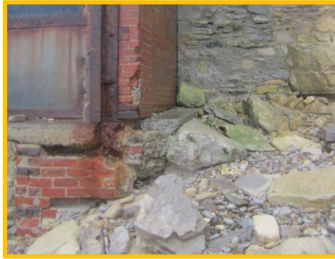
Undermining and loss of brickwork at north end of Redwell Land Lifeboat Stn.
