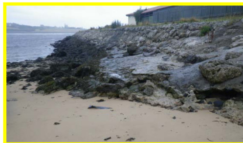
Erosion of mortar and loss of blocks at the toe of the wave basin revetment.
