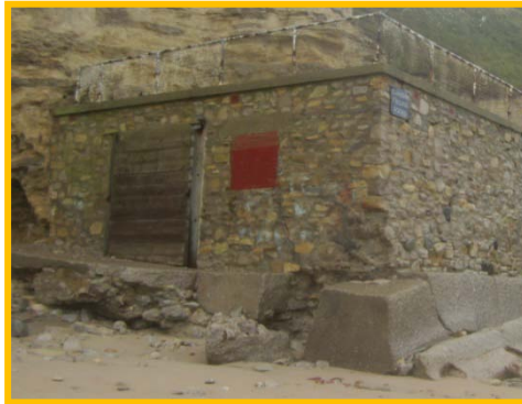
Undermining and displacement of toe beam and cracking in masonry wall.
