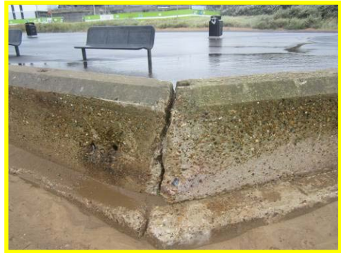
Cracks and spalling in low concrete capping wall.
