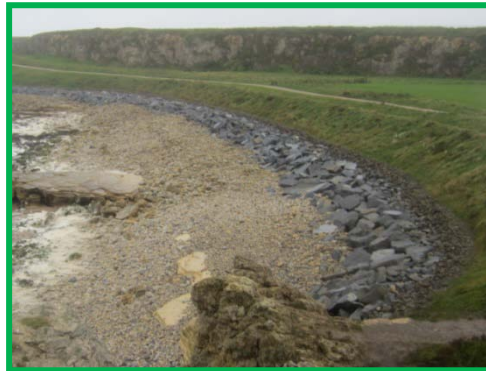
Rock revetment and grass slope at Graham's Bay in very good condition.
