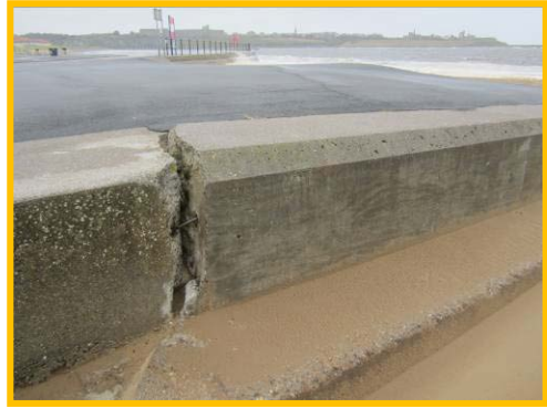
Settlement of the promontory area and wide cracks in the reinforced capping beam.
