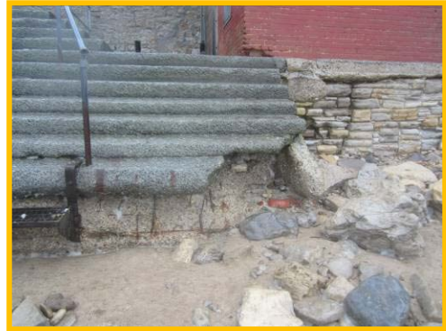
Undermining of stepped revetment and temporary metal access step.
