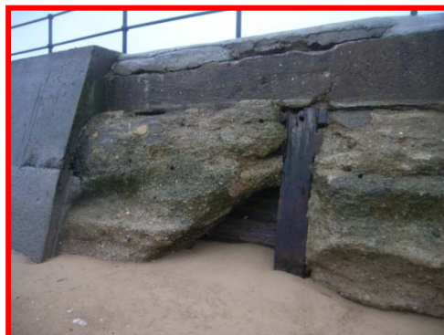
Failed front wall facing taken prior to storm on 24/09/12.
