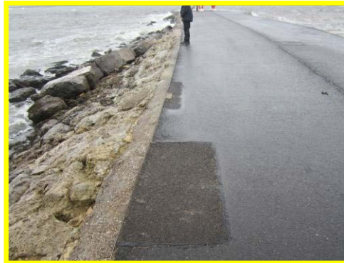
Repairs in asphalt surfacing to River Tyne South Groyne in good condition.
