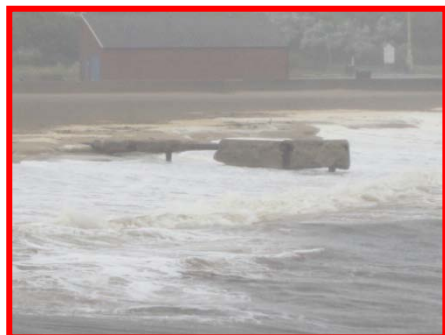
Obsolete outfall at Littlehaven
