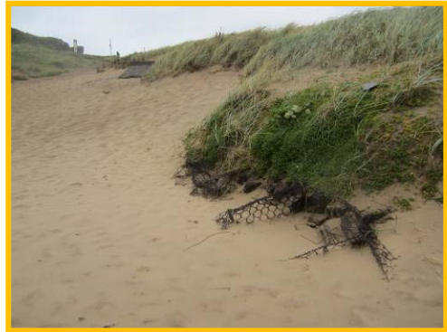
Exposed gabions at south (and north) end in poor condition.
