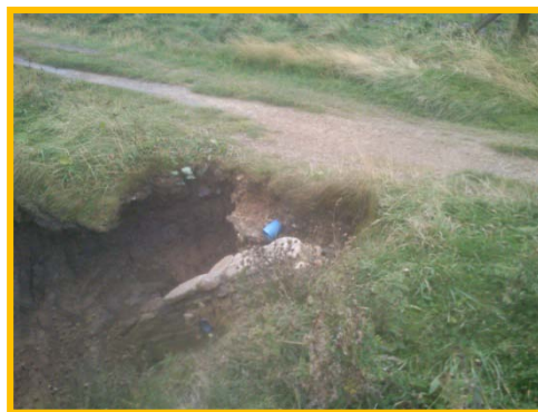
Localised erosion by land drainage outfall impinging on footpath.
