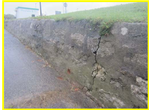
Vertical cracks in the retaining wall along the cliff top access steps.
