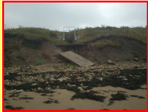
Failed scour apron at storm outfall in need of repair.
