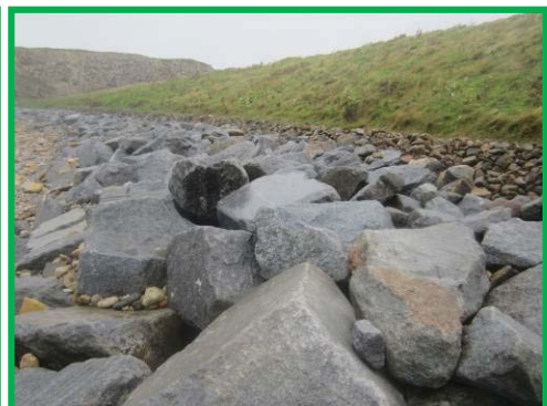
Rock armour stable and well interlocked with no erosion evident in earth slopes.
