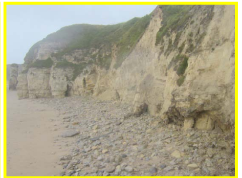
Small arches and caves in the base of the cliff south of the Lifeboat Stn.
