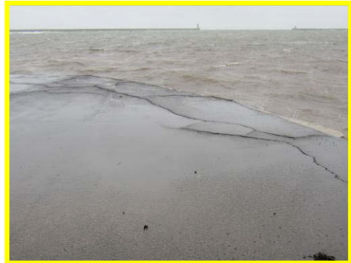
No significant change in cracks at seaward end since 2008.
