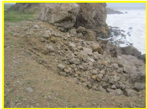
Ongoing erosion of loose rock slopes south of headland.
