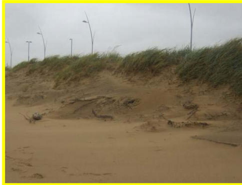
Some erosion along the toe of the dunes at the south end of Sandhaven
