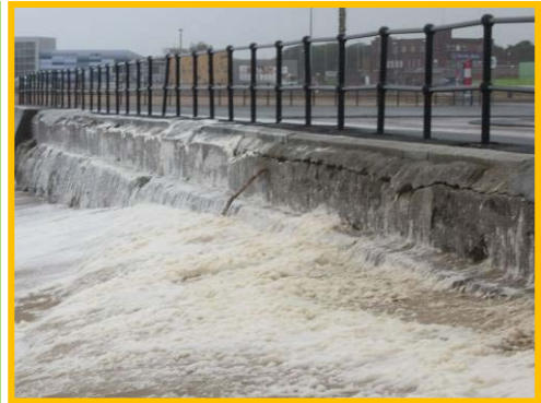
Cracks along concrete repairs at back of kerbing along the crest.
