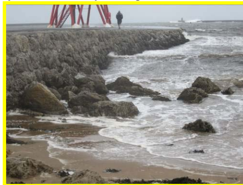
Movement of loosely placed rock armour along south face.
