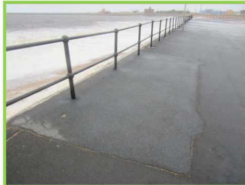
Repairs to surfacing due to overtopping damage still in good condition.
