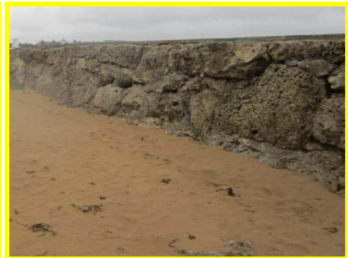
Void in concrete and some gaps between blocks along the south face.
